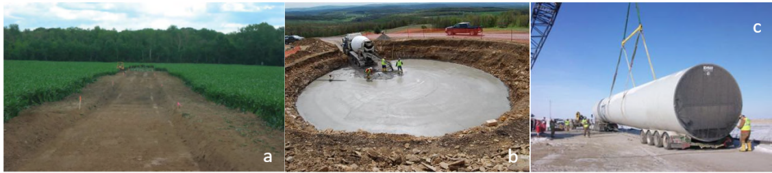
FIGURE 1.6: Activities of construction of a wind turbine (a. road construction, b. foundation placement, c. turbine erection).
